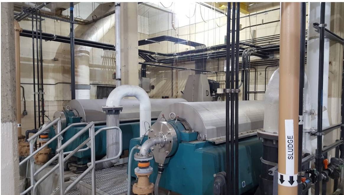
Centrifuges 1 and 2 at the Eastside WWTP
