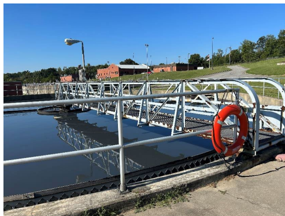
Example of a Primary Clarifier Bridge
