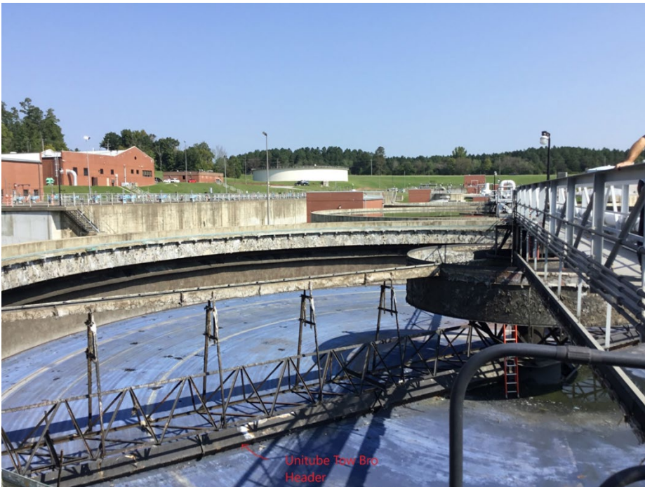
View of a drained final clarifier
