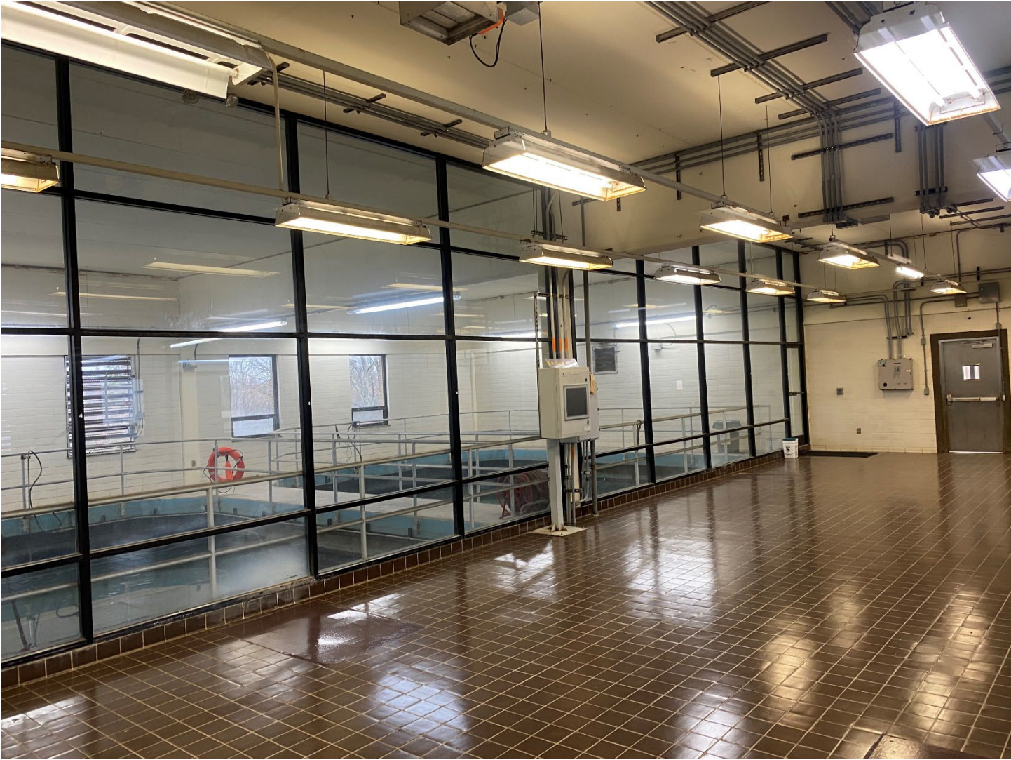
Ward WTP Filter Room
