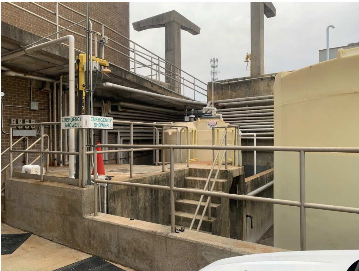
Chemical feed lines along chemical containment wall and water plant building
