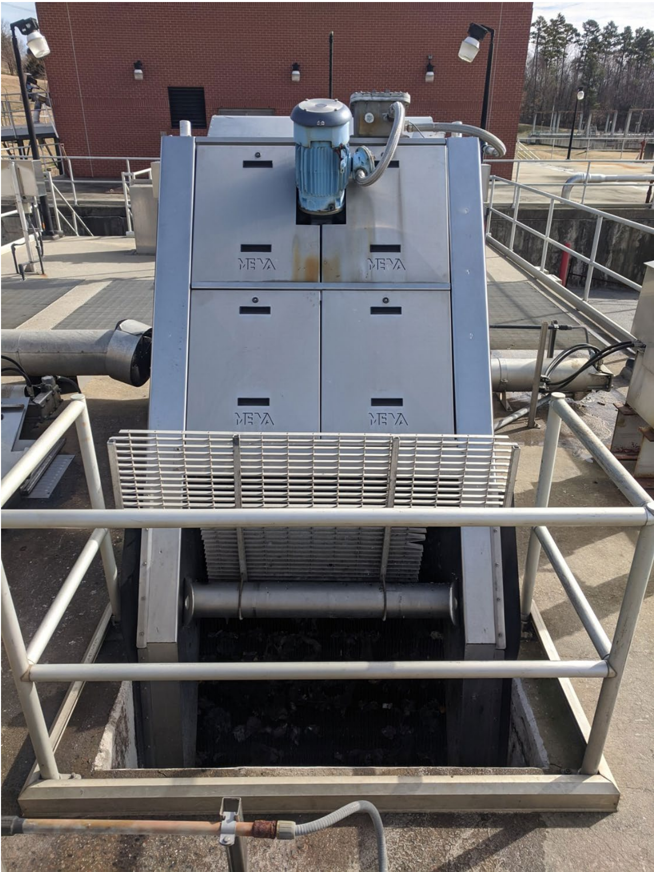
Example Bar Screen at the Eastside WWTP
