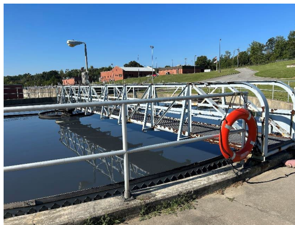
Example of a Primary Clarifier Bridge
