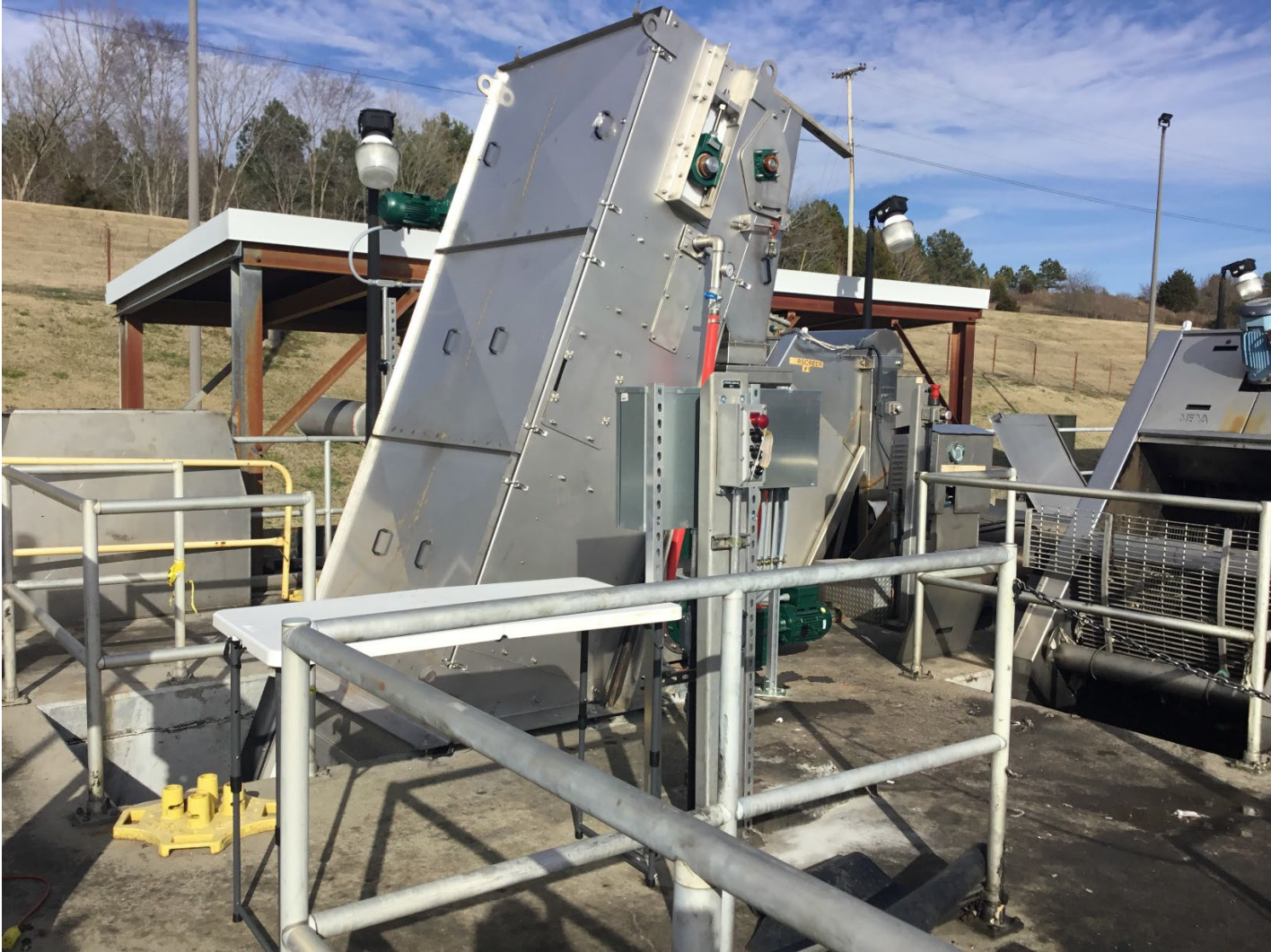
New Monster Fine Screen and Wash Press Eastside WWTP
