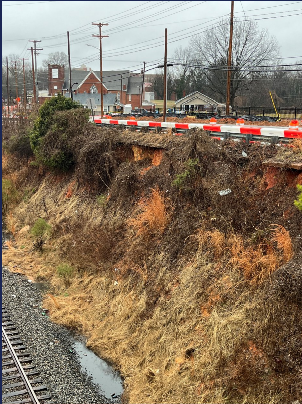
CURRENT SLOPE ISSUES ALONG WASHINGTON ST.
