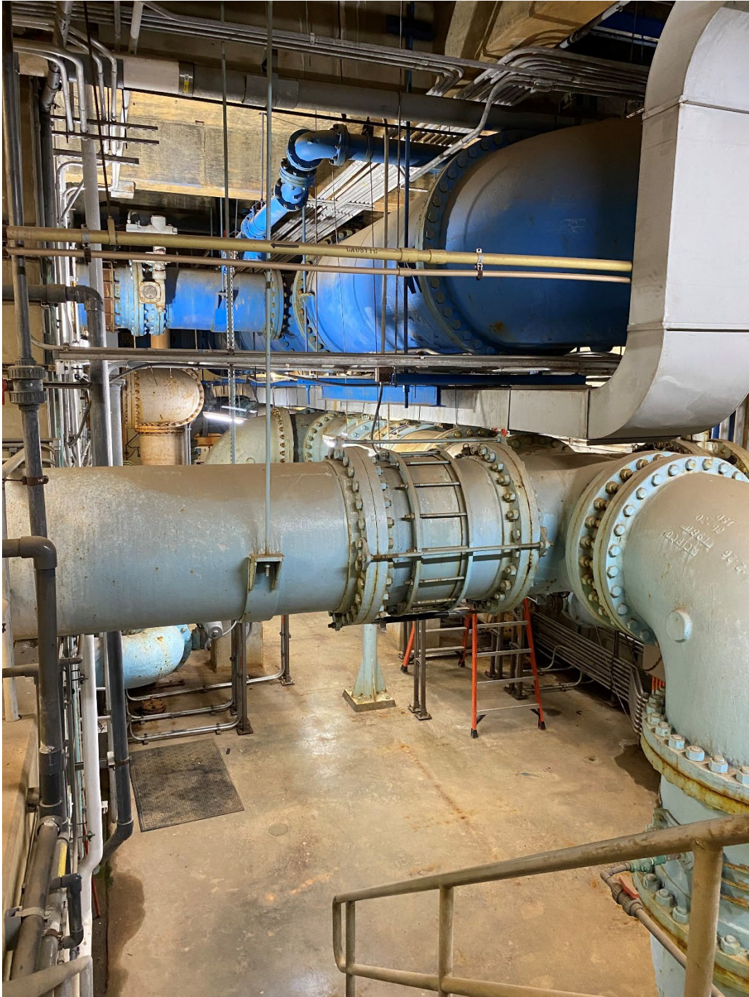
Ward WTP Pipe Gallery
