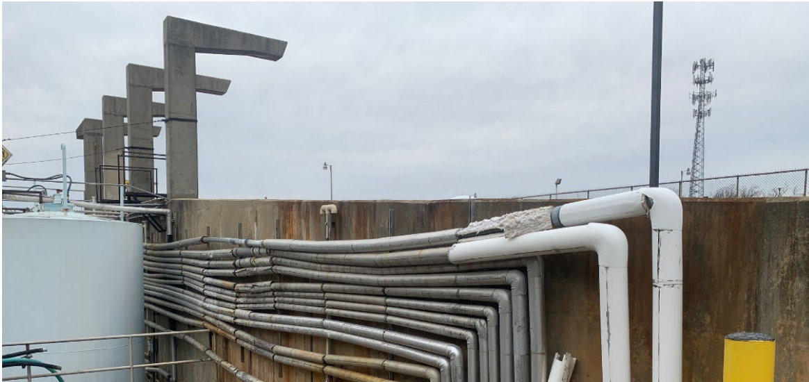
Chemical feed lines along the bulk chemical containment wall
