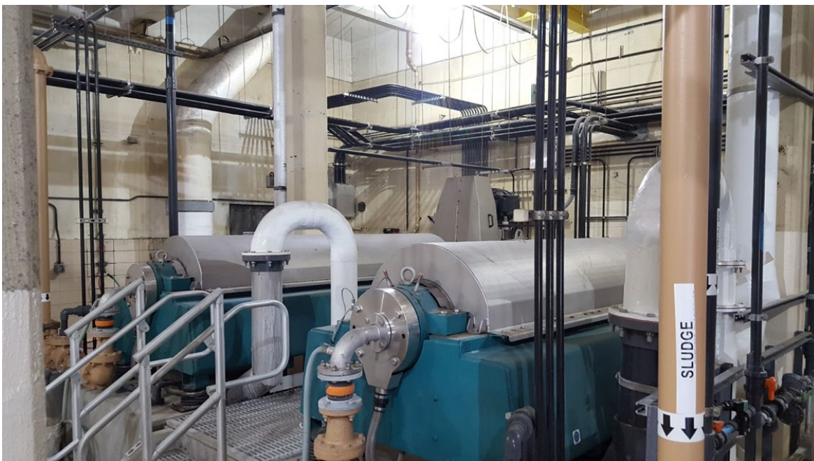
Centrifuges 1 and 2 at the Eastside WWTP
