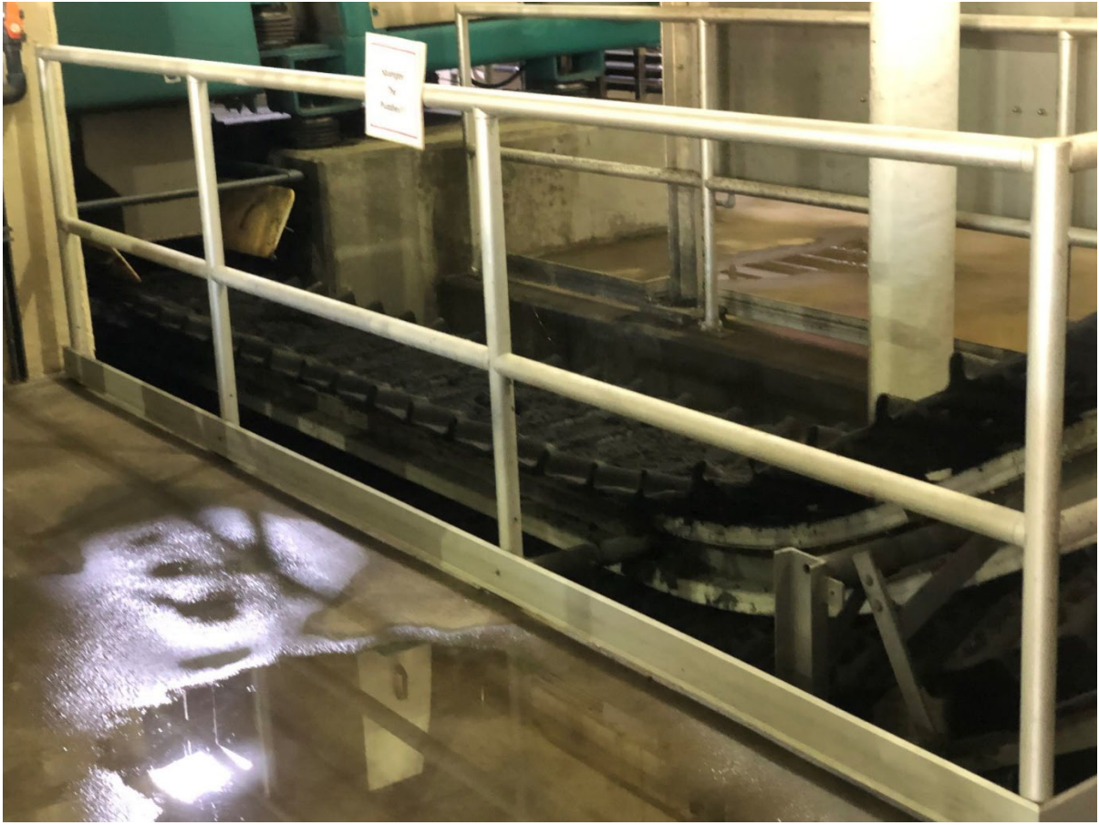
Serpentix Conveyor at the Eastside WWTP
