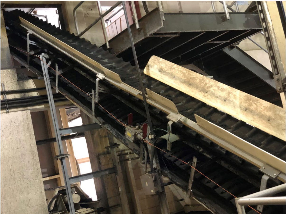
Serpentix Conveyor at the Eastside WWTP
